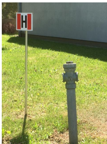
Hydrant na placu UTH
